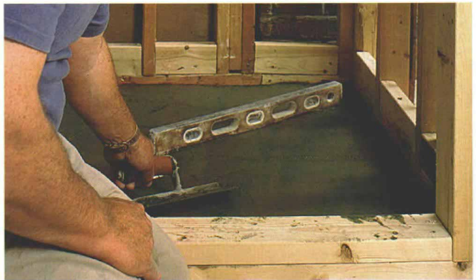
Getting the right slant. To build up the pitch on the pan floor, a fairly dry mix of 1 part portland cement to 3 or 4 parts sand is used to form the mud base (top photo). The mix should be just wet enough to form clumps when squeezed. Using a 2-ft. level as a gauge (bottom photo), the author floats a pitch of about 1/4 in. per ft. from the pan's perimeter to the drain.
